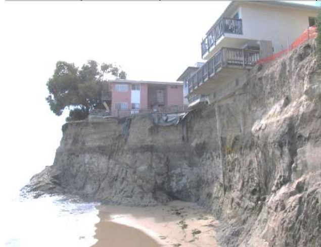
Figure 4. Cliff collapse at Isla Vista, California (taken 2005)
